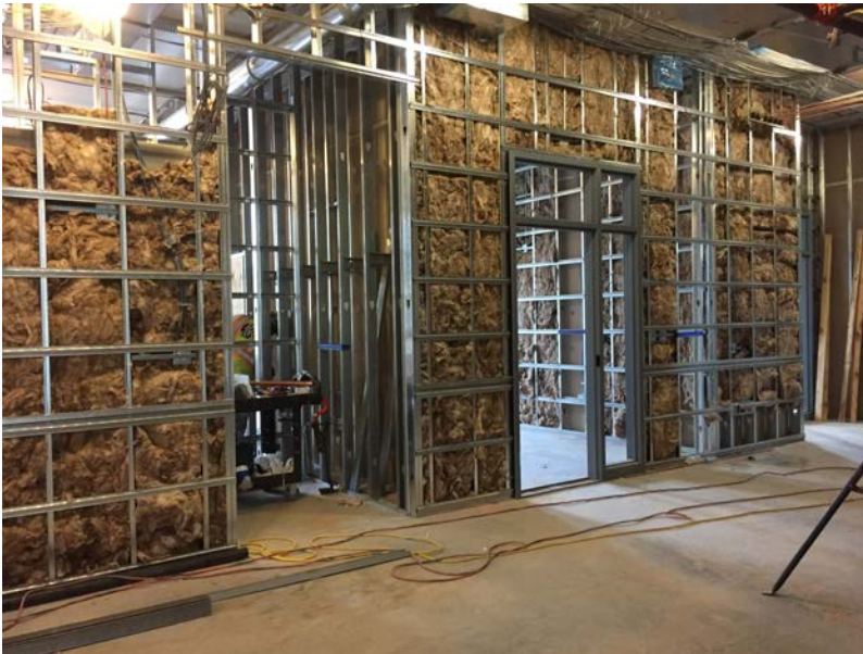
Framed walls and insulation on the second floor of the existing building
